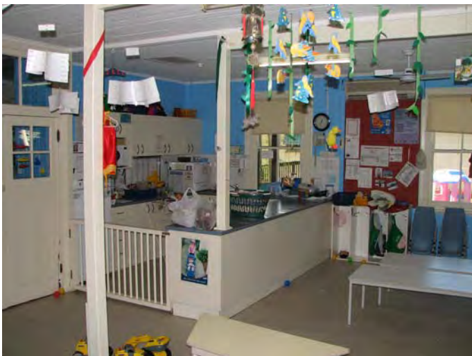
Plate 41: Block F. Modern joinery and other equipment has been fitted within the historic fabric, with adverse impact (JAA 2007)
