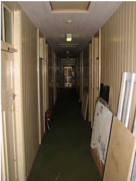
Plate 54: Block A. The central corridor extends the full length of the building. The timber walls, ceilings, door jambs, transom windows and timber trim are highly intact. This building is not one of the earliest Lennox House buildings, but lends itself to a high degree of conservation (JAA 2007)
