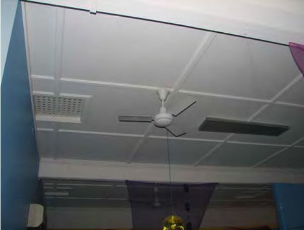
Plate 50: Block G. Dining room ceiling, with intact details including strapping and vents. These should be retained (JAA 2007)
