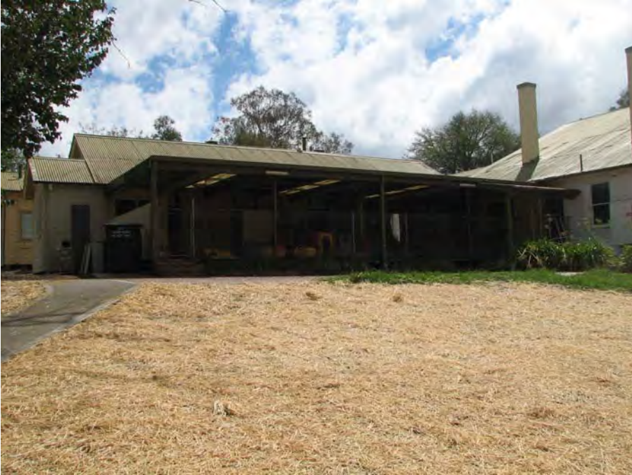
Plate 12: H Block; south-west side. The building is largely obscured by the covered deck (JAA 2007)
