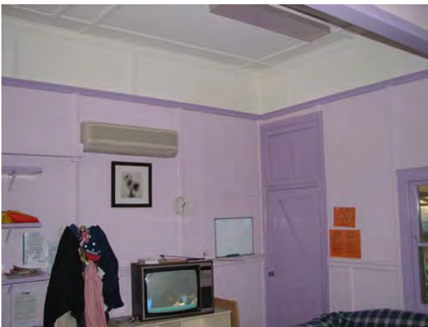
Plate 52: Block H. The staff room is formed by the removal of bedroom walls (see bulkhead above). Note the original braced and ledged door, picture rails, strapping and wall details. All of these elements are to be retained (JAA 2007)
