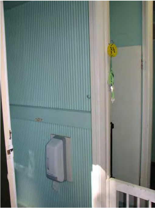
Plate 46: Block F. Ripple-iron toilet linings. These features must be conserved and retained (JAA 2007)
