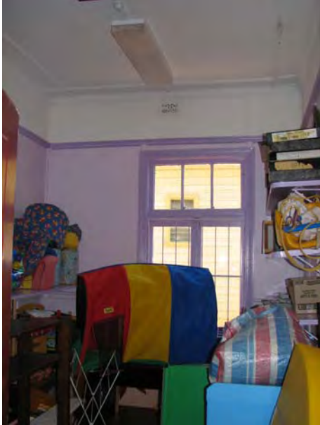
Plate 53: Block H. Store room with many original features of the building intact (JAA 2007)
