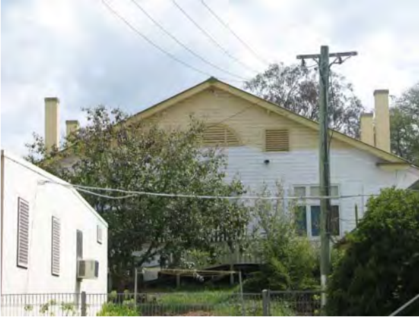
Plate 36: Block G; east façade. This was added in the 1920s, with little regard for the original symmetrical façade (JAA 2007)
