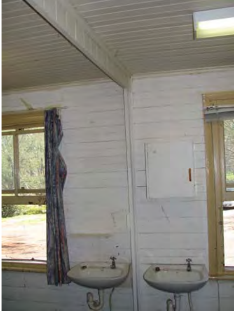
Plate 55: Block A. A wall separating two original bedrooms has been removed, but a bulkhead and nibs have been retained to identify the earliest arrangement. All bedrooms had basins, but those in the picture are not original (JAA 2007)
