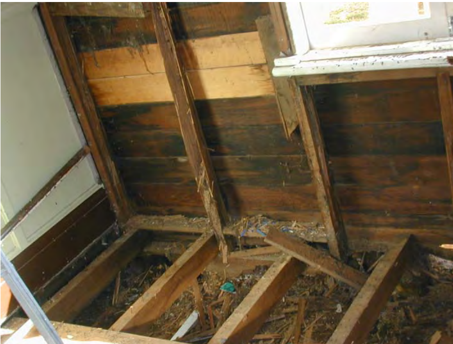
Plate 24: Block D – damages as a result of termite infestation (JAA 1998)
