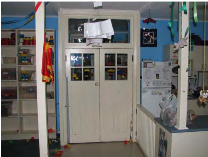
Plate 40: Block F. original doors and other joinery details survive aside the colourful presence of child-care activity (JAA 2007)
