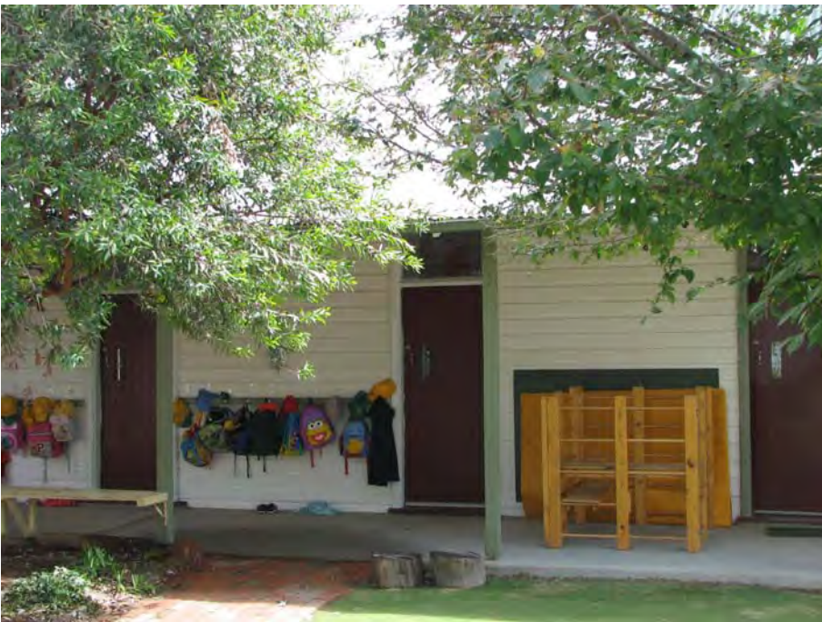
Plate 5: D Block; east side. The HMP recommends replacement of the concrete floor and posts (JAA 2007)
