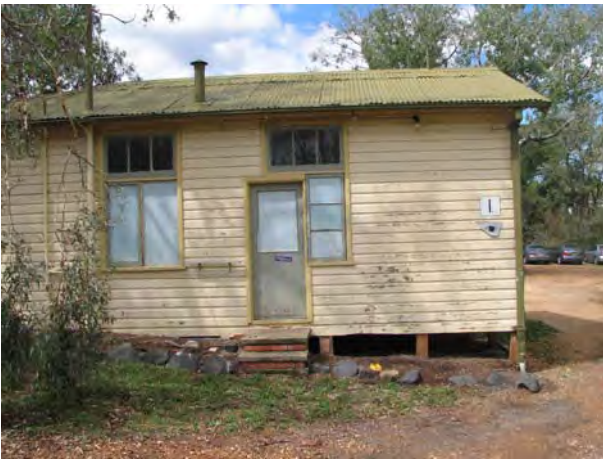
Plate 34: Block I; west end. Note the crude installation of the door into the partly demolished window (JAA 2007)
