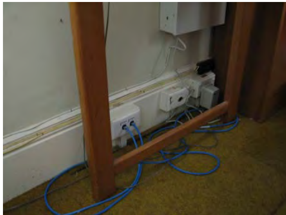
Figure 4.34: Damages and poor installation of services in the cottage at 7 Liversidge Street.
