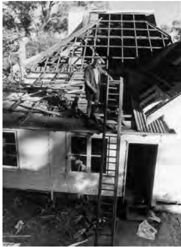
The demolition of Cottage #2 to make way for the Acton Tunnel (ACT Heritage Library. Ref 003729)
