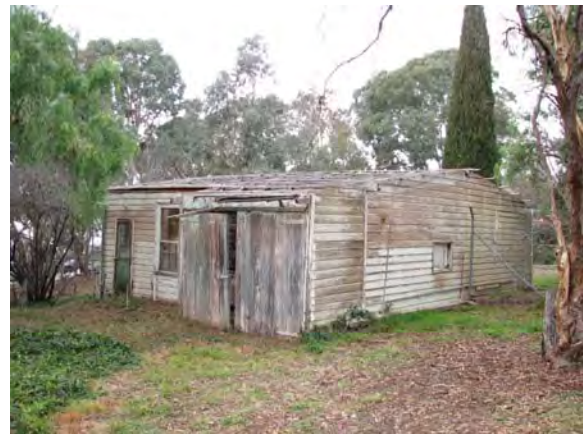
Figure 4.30: The intact laundry and loose-box buildings, and dilapidated stables/garage at 16 Lennox Crossing, 2009.
